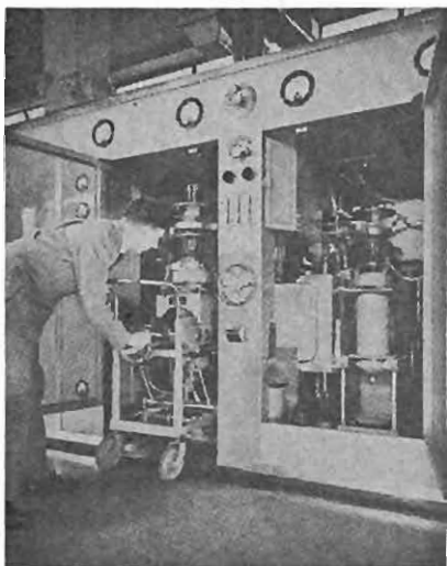
Changing tubes in a big transmitter is no easy task. Here we see an engineer at Daventry (England) wheeling a 112 pound water-cooled tube into place. Owing to their enormous size, these tubes are always moved on the small trolley, which has a special device for fitting them into position in the transmitter. (Courtesy of the British Broadcasting Corp.).
